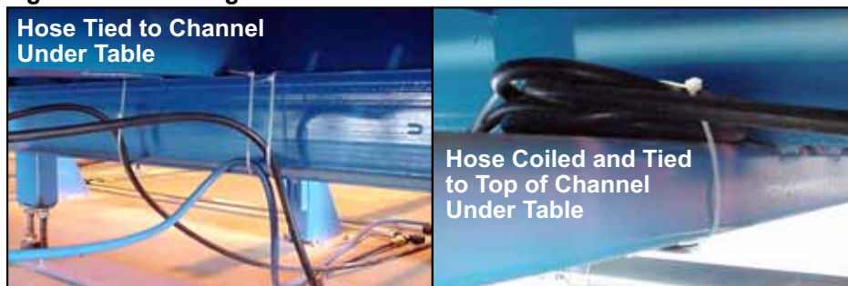
Figure 5-1: Securing Hoses Off Floor
