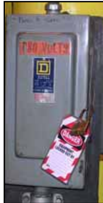
Figure 2-3: Sample of a Lockout/Tagout Mechanism on a Power Source Panel
